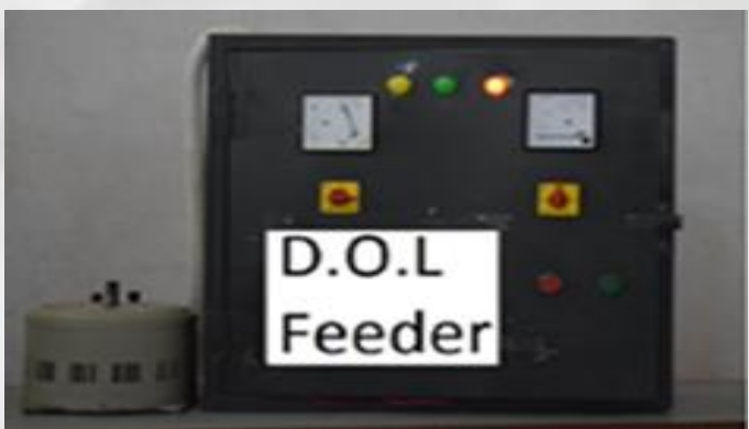
Industrial Standard Induction Motor Starter Panel For Reverse And Forward Rotation Operation
