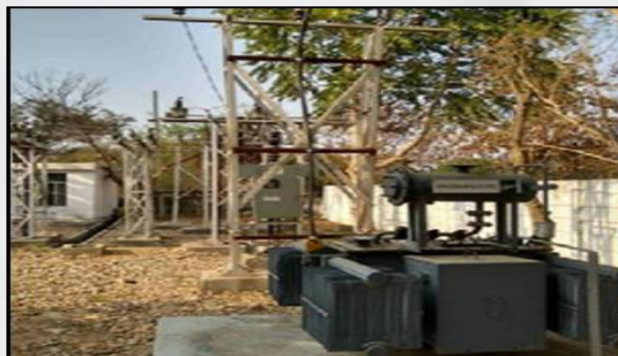
Industrial Standard Transformer
